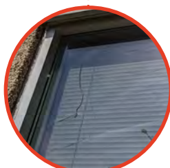
Aluminum Frame with Cracked Glass
